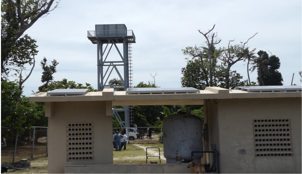
The new Kayangel State Solar-PV water pumping and supply system, has replaced the electric motor driven pumps of the Kayangel well water systems helping to enable all residents to have water. (photo by S. Abraham(SPREP))
